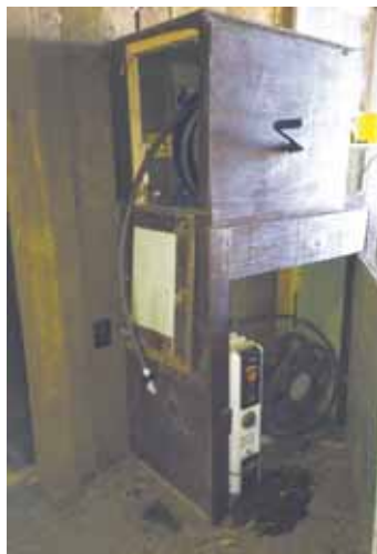
Heated hose box is mounted to an outside wall and plumbed into barn's bathroom. Radiator-type space heater at bottom keeps hose warm all winter.
