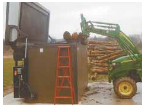
Big firebox on Tom Lubbers's top loading wood boiler holds up to 1 3/4 cords of wood, in chunks up to 9 ft. long.
