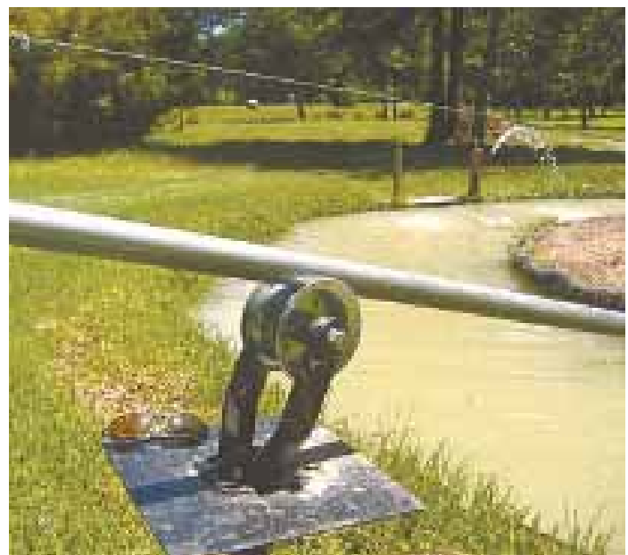
Pipe rides on a small metal roller mounted on a pedestal base.
