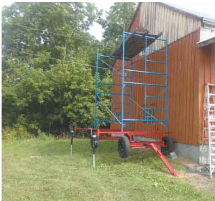
Scaffold is mounted on running gear off a 3-ton hay wagon. Leveling jacks at bottom can be telescoped in or out to keep scaffold level on uneven ground.
