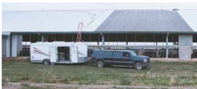
As Schmidt lowers washer down roof's steel ribs, it leaves an obvious white path next to unwashed grey metal.
