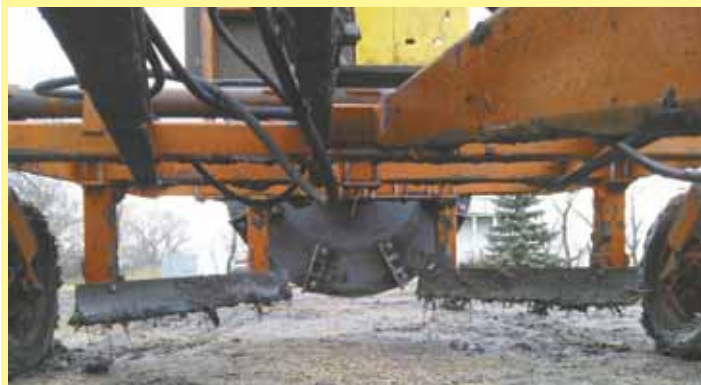
A pair of steel gathering blades under frame move dirt toward the center, which results in a wider cut than just the radius of the cutting wheel.
