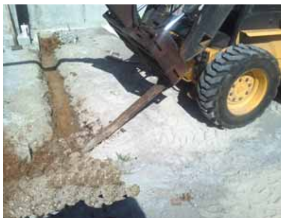
Matthew McKinzie uses a single skid steer pallet fork to dig narrow trenches. "I just slide the fork into the ground at an angle and rotate it up," he says.
