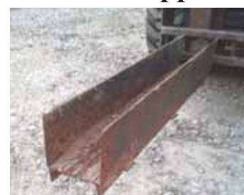
McKinzie cut a piece of channel iron to fit over the fork and uses it to clean loose dirt out of trenches made by fork.
