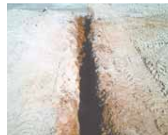
He uses the same idea to loosen rocks, roots and dirt so he can get in with a bucket later to scoop out the material.
