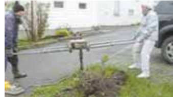
Posts can be driven into ground by hand or with a 2-man power driver.
