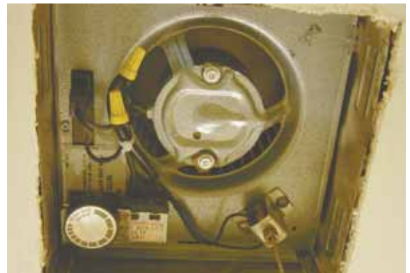
Kiefer installed a humidistat from an old dehumidifier (lower left) and a pull switch (lower right) to his bathroom fan.
