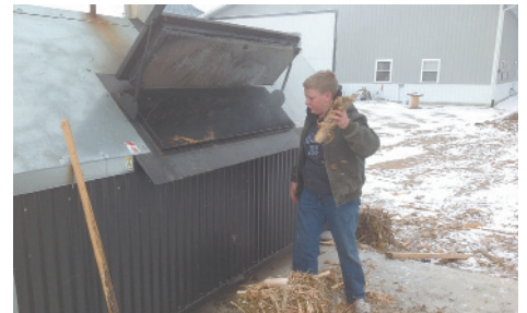
Adlai is shown here feeding the fire in their Log Boss wood-fired boiler. The Miscanthus grass burns hot and clean.
