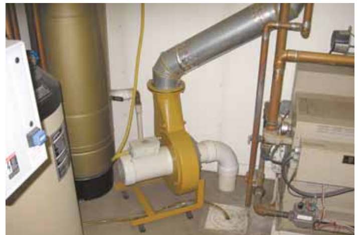
A blower fan pulls exhaust through the pvc pipes under shop floor and expels it outside of building.
