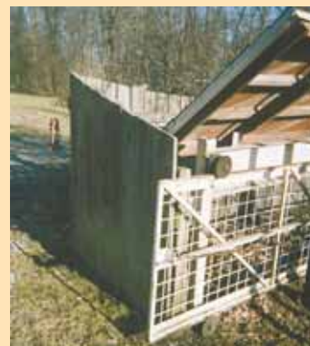
Linnemeier pieced livestock fencing panels together to build the 24-ft. long gate.
