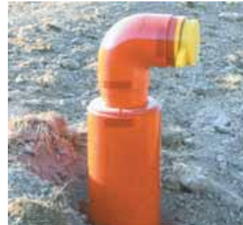
A dry fire hydrant is a non-pressurized pipe system with one end in water and the other on dry land, where a pumper truck can access it.
