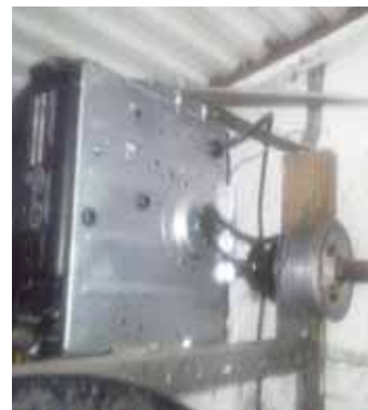
Needing more overhead room in his garage, Dan Eagleton converted the garage door opener into a side-mounted one.
