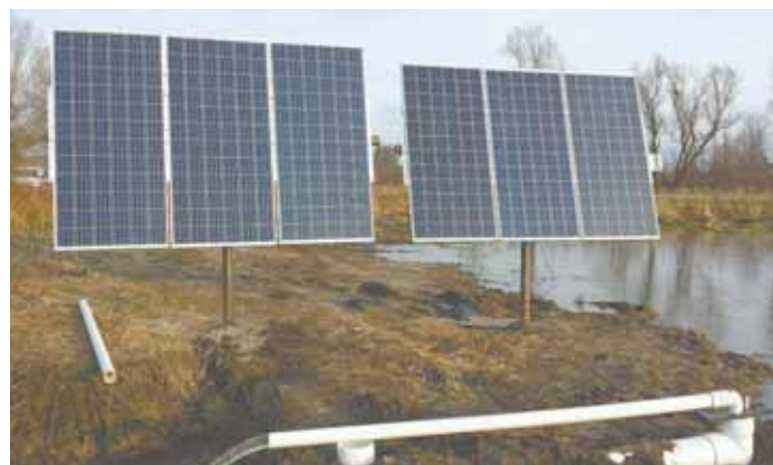
Jamie Near designs solar systems that power pumps to drain tile in remote fields. "Solar makes sense when grid power is 1/4 to 1/2 mile away or farther," he says.
