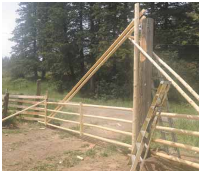
"It's a lot of work to build a gate like this. But it's eye catching and a lot of people marvel at it," says Bill White about his timber "pole gates".
