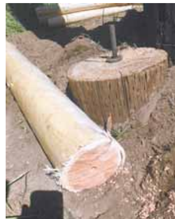
Gate's hinge pole swivels on a short length of rebar mounted vertically in center of a 2-ft. section of telephone pole that's buried in the ground.
