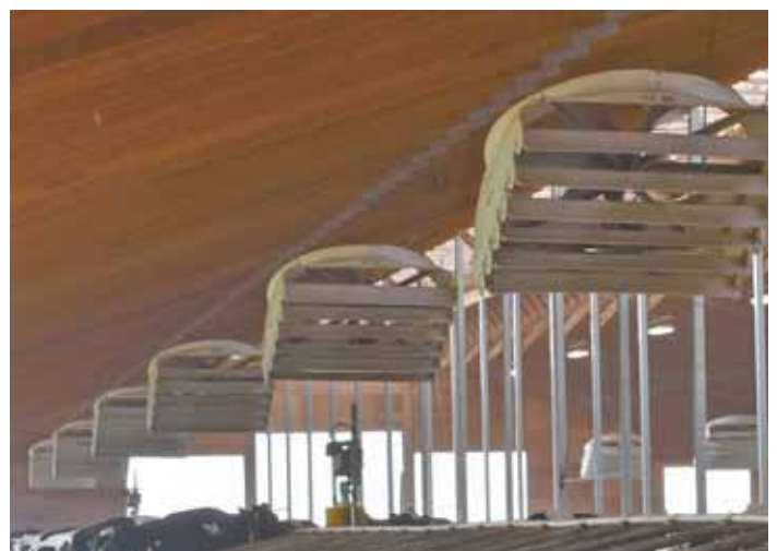
High velocity Storm fans from Barn Solutions come with adjustable louvers that let you direct the air over and under cows, or around obstacles.
