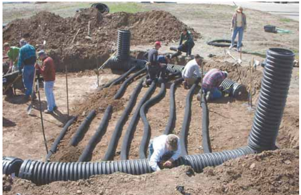
Climate Battery blows hot, humid air through pipes and into the cool soil beneath a greenhouse, where heat and humidity are released. By the time the air returns to the greenhouse it’s cooler and drier.
