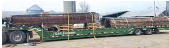
Two 40 by 100-ft. buildings were torn down and loaded onto this semi trailer, ready to be re-erected.
