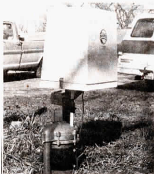
Chlorinator mounts on the well-head and drops chlorine pellets directly into discharge point.
