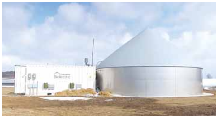
Mini digester can produce electricity from herds as small as 75 head or less. It produces biogas that fuels an internal combustion engine attached to a generator.
