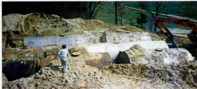
Tanks are staggered in three rows and set back into side of hill.
