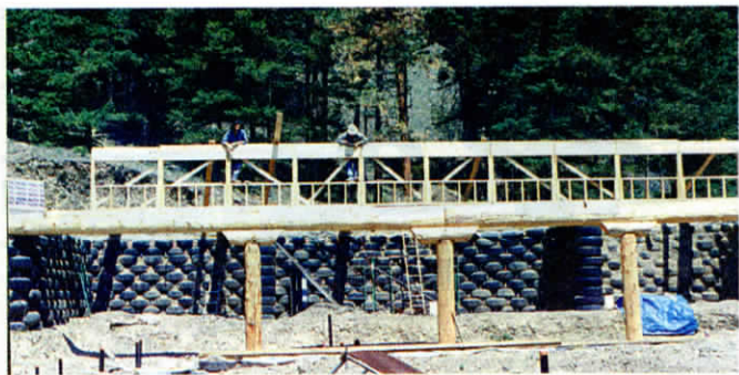
Old tires are formed into 350-lb. "bricks". The tremendous weight of a wall made of tire bricks makes cement foundation unnecessary.
