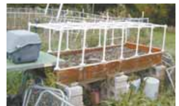
He made another bed by stacking concrete blocks under a steel door with sides made out of old 2 by 8s.
