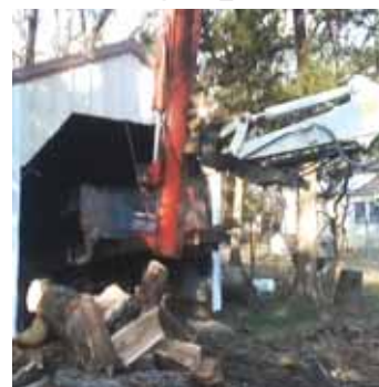
Log splitter mounts in place of the bucket on Zimmerman's compact excavator.
