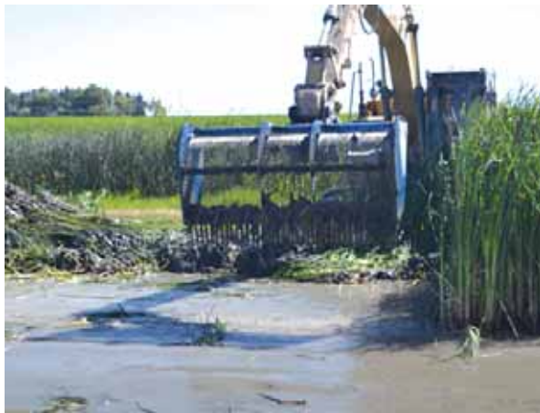
Teeth on big bucket rake allow water and silt to drain through while capturing vegetation and floating debris.
