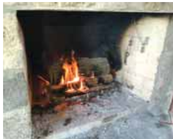
Fireplace grate made from black pipe takes heat from upstairs and sends it down to Reinholm’s basement using a small 3-speed recirculating pump.
