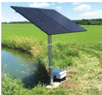
Solar aeration works well for ponds without access to power.
