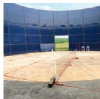
An old 20-ft tall by 52-ft. dia. Slurrystore was cleaned up and converted into a pickleball court.
