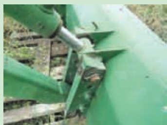
New pins were made from 4140 bar stock and the cylinder seals were re-packed and fitted with new hoses and connectors.
