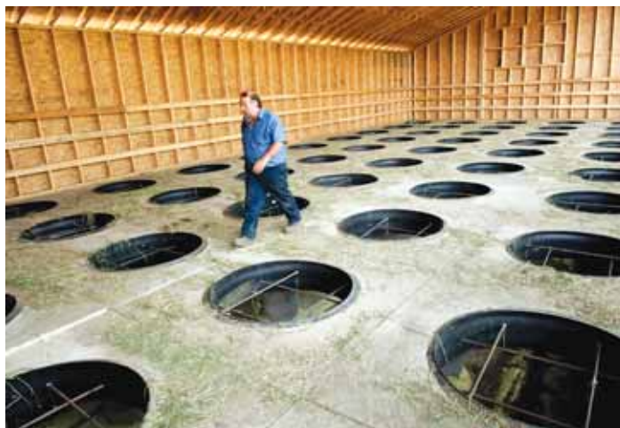
A concrete floor, with holes sized for the 5-ft. bales, holds the hay as it’s brought from the fields. Metal grating in each floor opening supports the bales above 4-ft. deep insulated ducting.
