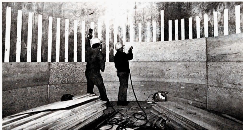
Crews essentially build a barrel inside the silo by nailing 1 by 4's directly onto silo walls, then stapling on ¼ in. plywood liner. Base price for converting a 20 ft. dia. silo is right at 35 cents per bu.
