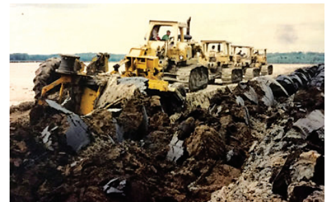
It took four D8 and D9 Caterpillar dozers linked together with cables and chains to pull the plow.
