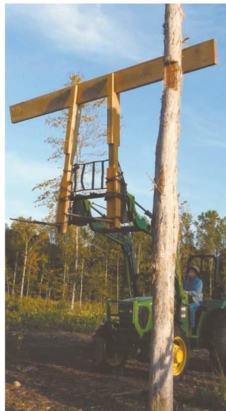
Agnew uses home-built loader-mounted truss lifter to raise wood beams up to 20 ft. high, then bolts them into notches cut into building’s posts.
