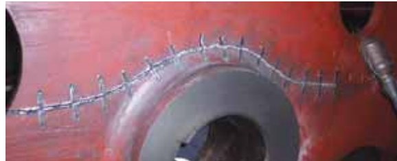
Metal stitching can repair cracked or broken cast iron, creating a part that’s stronger than the original.
