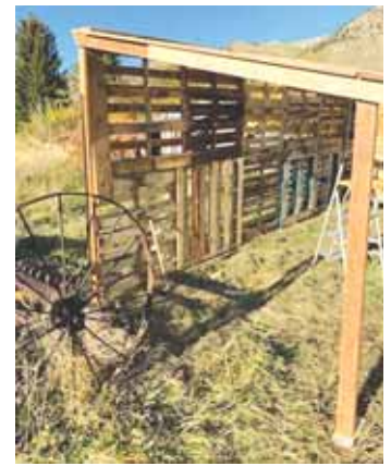
Miller built a low cost structure using pallets, steel posts, used 2 by 4's and some billboard tarps.
