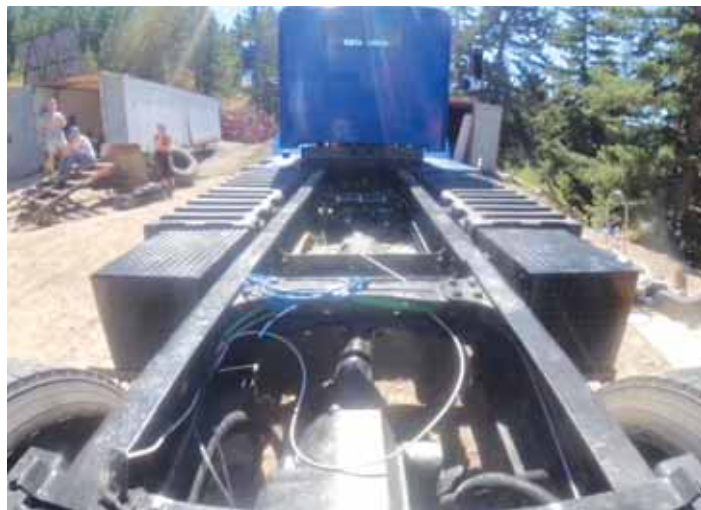
Retrofit Kenworth battery modules to side of frame rails.
