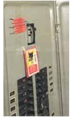
After a friend had a fire that started in her breaker box, Hutson taped firecrackers next to his circuit breakers.
