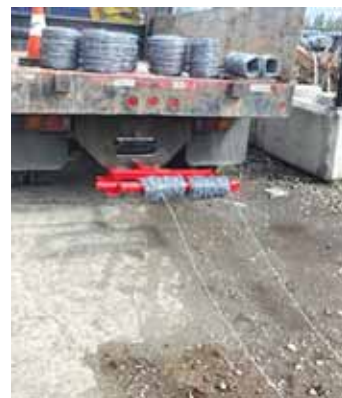
Wire holder welded from tube steel and angle iron allows wire to unwind.
