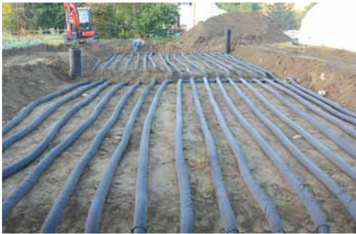
Perforated drain tile with a sock inserted into lower holes of manifolds.
