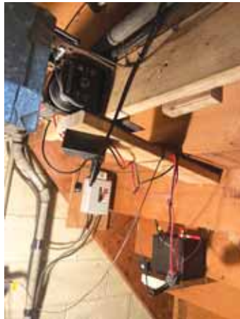
Lift battery and winch under stairs.
