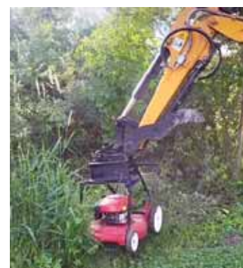
Carolla's "flying lawnmower" attached to his Sany mini-excavator works great for trimming grass in hard-to-reach places like ditch banks and around ponds.
