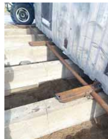
Steel skids were constructed of 4 by 6-in. steel tubing laid on top of concrete pillars and welded in place as spreaders.
