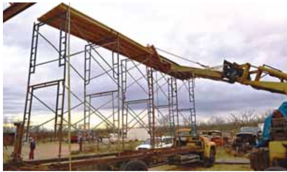
18-ft. tall bus chassis scaffolding with a 24-ft. platform on top provided a stable work platform for Surber to install the trusses for his shop.
