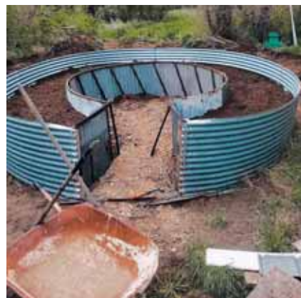
Taylor used the bottom ring of a damaged 14-ft. grain bin as a raised garden bed.
