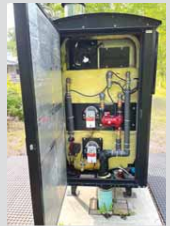
Hohl’s “best buy” Heatmaster G4000 outdoor wood boiler sits on an insulated cement pad.
