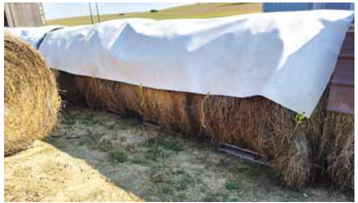
Evensberger bought the membrane and added tarp grommets spaced every 4 ft. around the bales to keep the TPO down.
