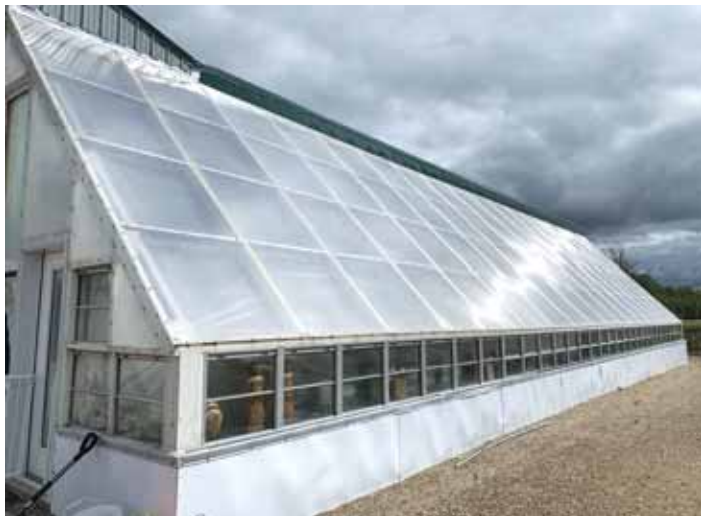
The south face consists of glazed 8-mm twin wall polycarbonate placed on 2 by 6-in. framing with the glass glazed only where the sun hits.
