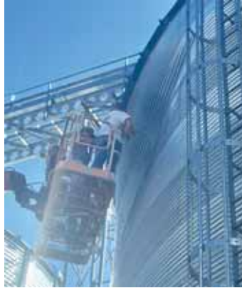
Build Summit repairs grain bins by removing dents and replacing sheets as needed.
