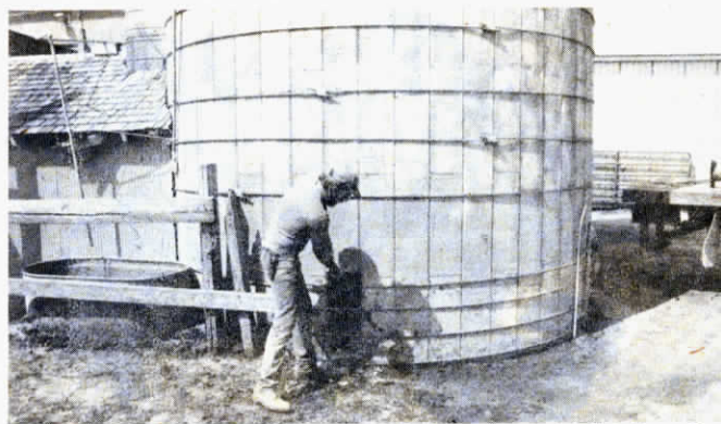
Dave Carpenter is shown knocking out a couple of staves to create a hole for pulling out the silo unloader with a skid steer loader.
