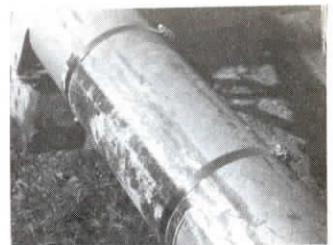
Patch simply fits in place over damaged area with two screw-tightened clamps.
