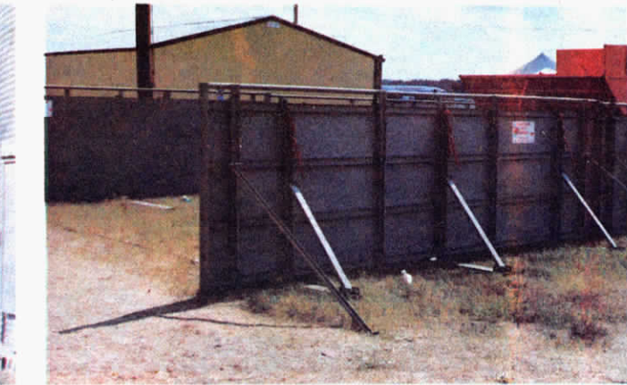
Stabilizing chains keep the side panels from moving apart once the bunk is filled with silage.
